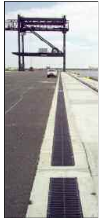
Port Trench Drain
